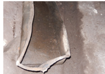
Damaged rubber boots
