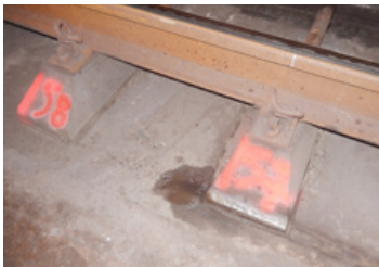
Water ingress old booted block
