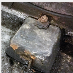
Damaged booted blocks
