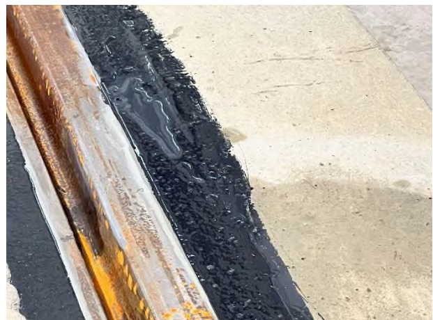
Fig. 3 - Residual water on the joint sealant
